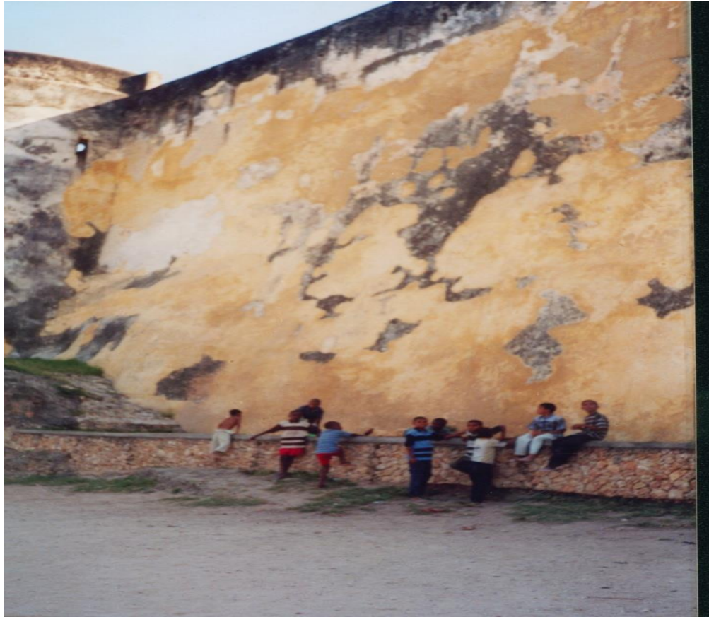
Plate 6.8: Outside Patched Wall of Fort Jesus (Source: NMK, 2011)
