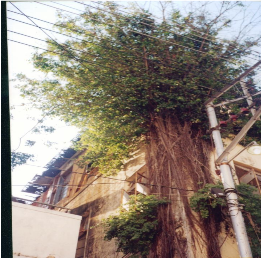
Plate 6.10: Tree Growing On the Wall in the Old town just opposite Fort Jesus.(Source NMK, 2010)
