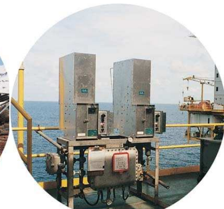
Off shore: 200 watts communications and safety equipment, multiple systems - Thailand
