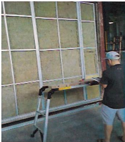
Plate 1. Before the test. (during the construction showing the rockwool infilled and studs)
