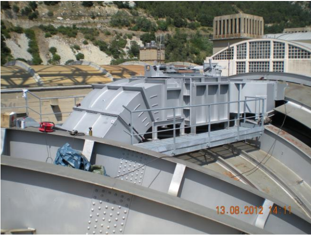
EAR inlet circuit mounted without its shelter.
