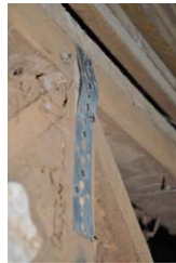
(g) GUA 390%: Connection– Location 7: South transv.wall
