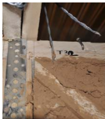
(j) GUA 390%: Ligature wire–Location 8: West shear wall
