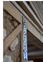
(e) HTI 300%: Connection–Location 7: South transv. wall
