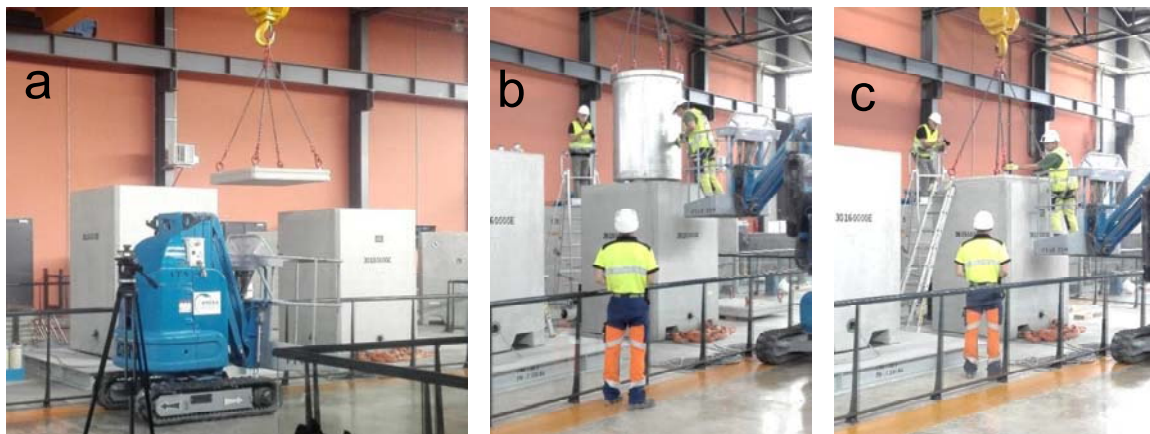
Figure 3. General overview and handling of the dummy primary waste package, a) remove the lid, b) loading the container with a dummy primary waste package, and c) closing of the waste package
