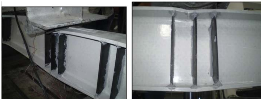
Fig. 9. Local cracks in T1_1.
