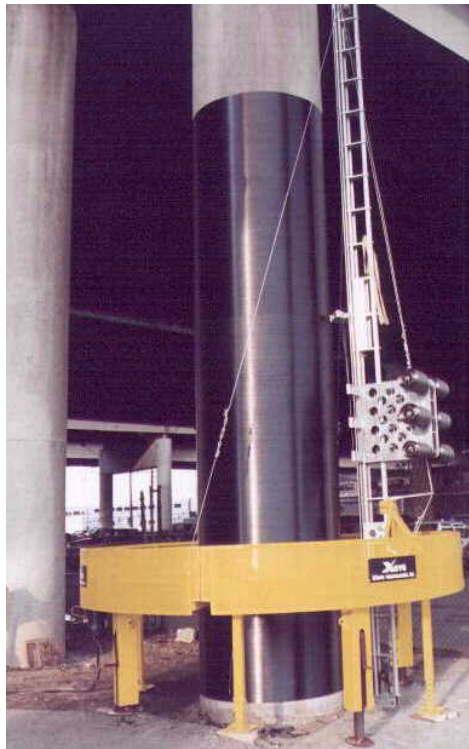
Figure I.2. 8: Procédé de l'enroulement filamentaire (Master Builders, Inc. and Structural Preservation Systems 1998, Balaguru et al. 2009)
