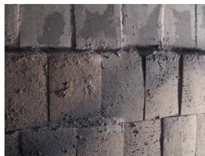
Figure 1: New (top) and old (bottom) SiC based refractory tiles (oxides binders) in a WTE facility (tile height: 245mm)
