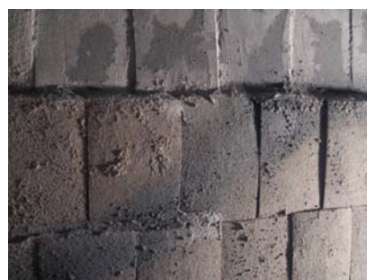
Figure 1: New (top) and old (bottom) SiC based refractory tiles (oxides binders) in a WTE facility (tile height: 245mm)
