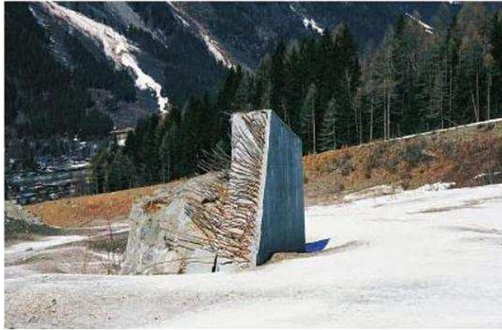
FIGURE 2. Protecting wall in armed concrete at Tacconnaz (Haute-Savoie, France) destroyed by the powder-snow avalanche of the 11 February 1999. The height is 7 m and the thickness is 1.5 m (Photo by C. Ancey).
